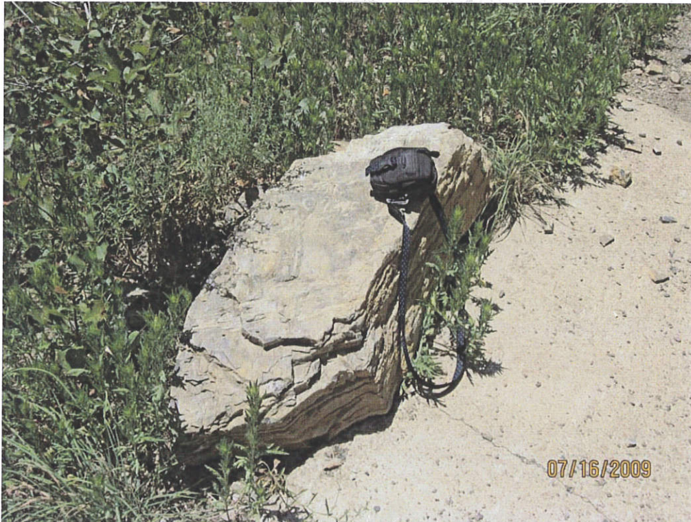
Another large rock from recent rock fall on Ogden Canyon Canal Conduit
