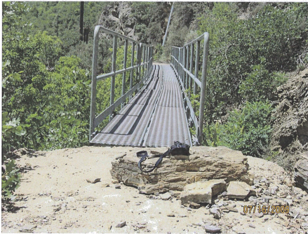
Large rock from recent rock fall on Ogden Canyon Canal Conduit
