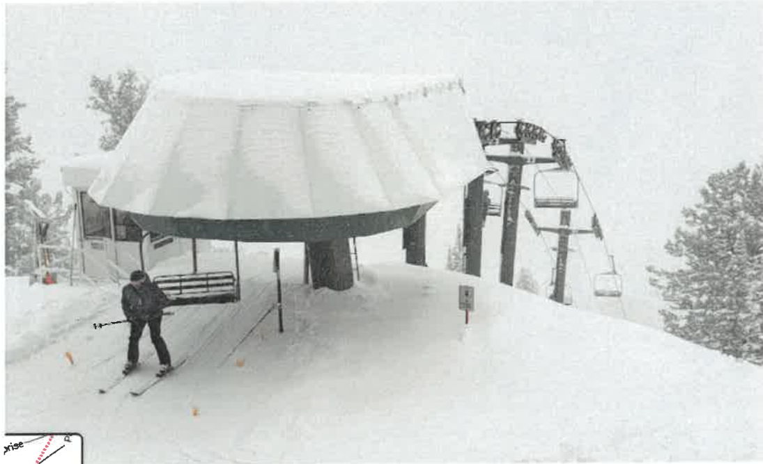
Current lift terminal near Needles Lodge, at the top of Middle Bowl.
