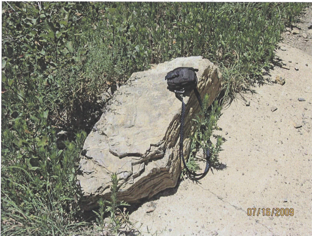
Another large rock from recent rock fall on Ogden Canyon Canal Conduit
