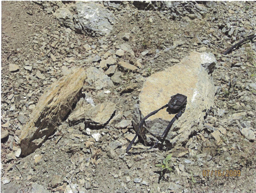
Possible rock fall on the central portion of property
