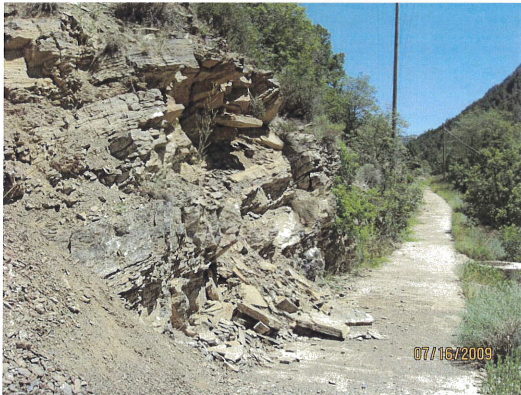
Small rock fall on Ogden Canyon Canal Conduit Road
