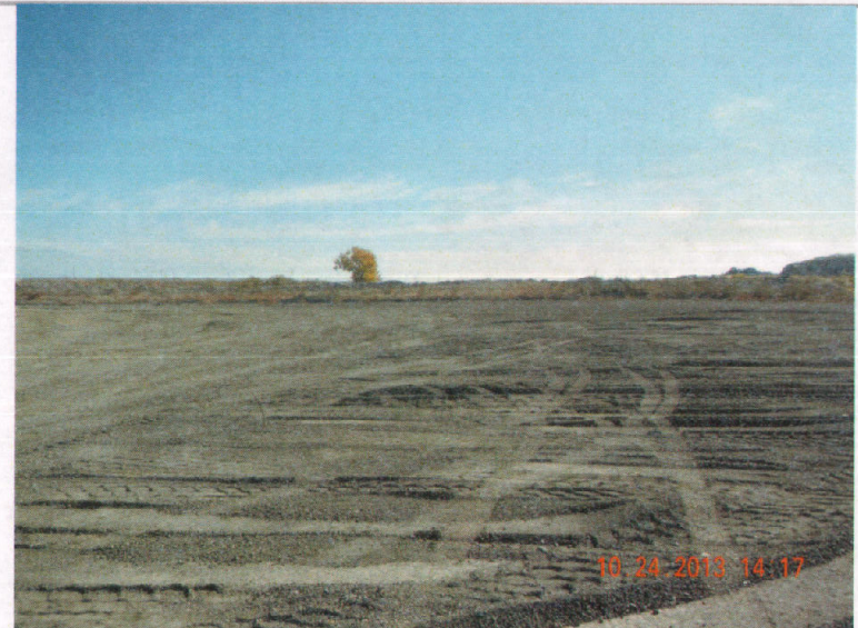
View from center of site to the southeast with topsoil perimeter berms and heavily trafficked flat area.
