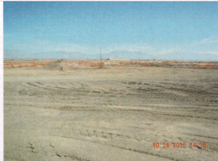
Disturbed flat area with remaining gravel piles and perimeter topsoil berms
