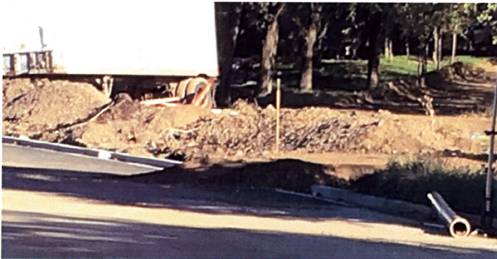
Needs to be a pipe under the dirt in the gutter so water can flow down the gutter
