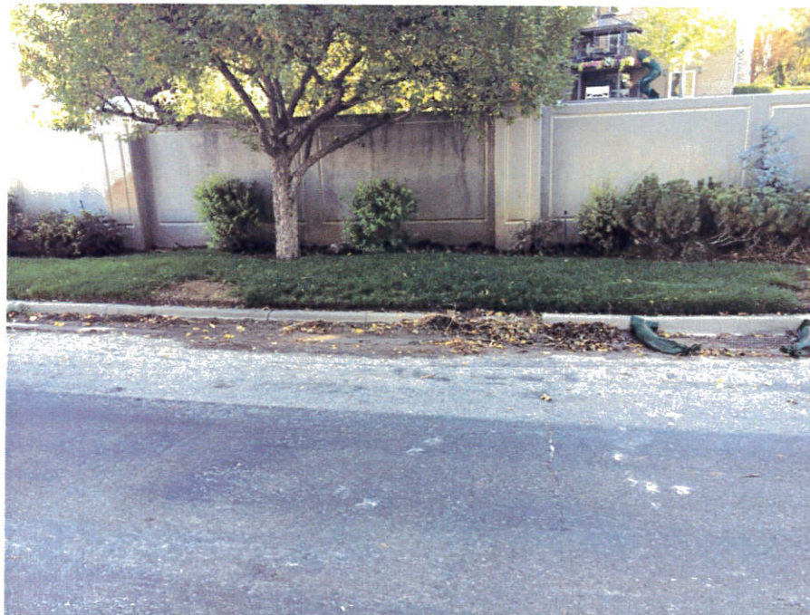
All catch basin BMP's need maintenance
