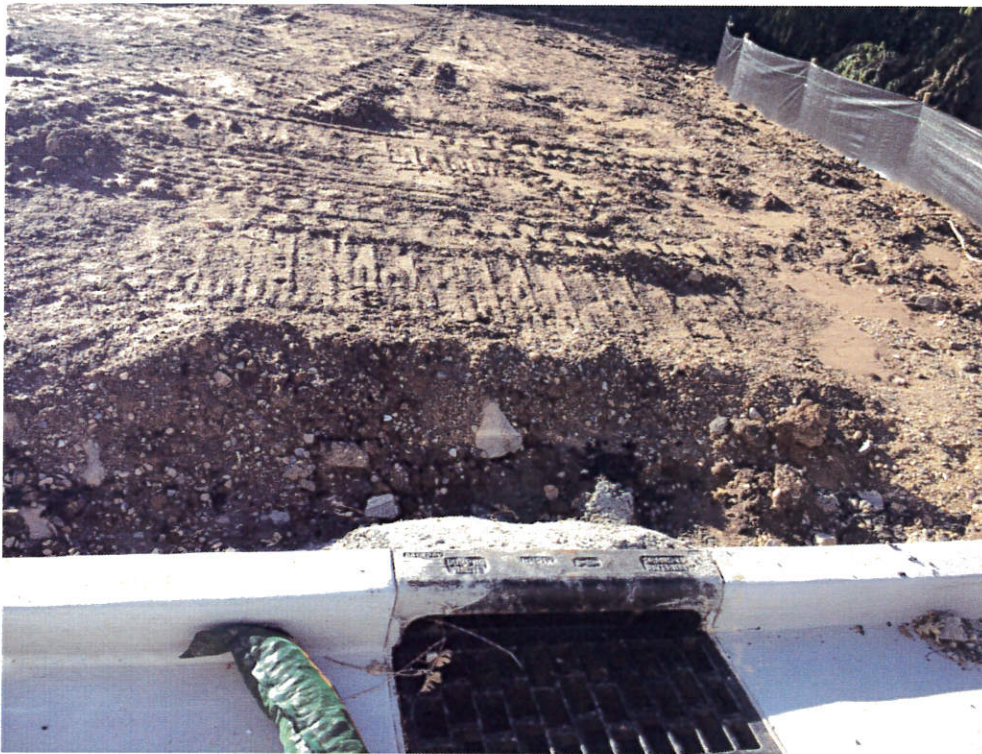
Disturbed areas are eroding and require final stabilization measures to be implemented ASAP
