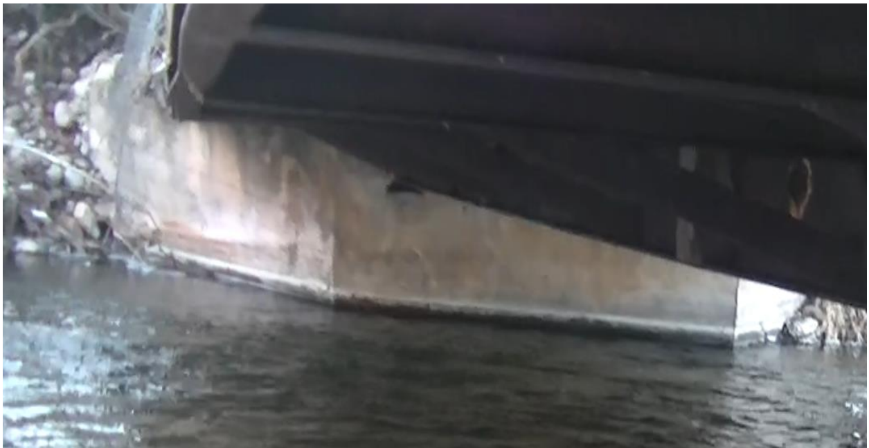
Figure 7. Post-flooding and repair photograph of northwest bridge abutment.
