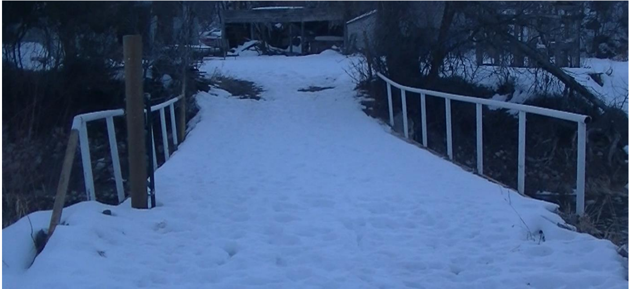
Figure 4. Bridge condition on January 1, 2024 looking west (after 2023 flooding and bridge repair).
