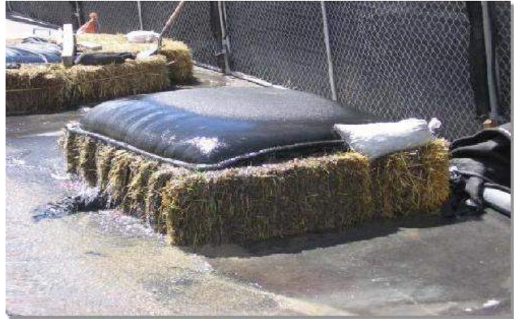
Photograph DW-1. A relatively small dewatering operation using straw bales and a dewatering bag.
