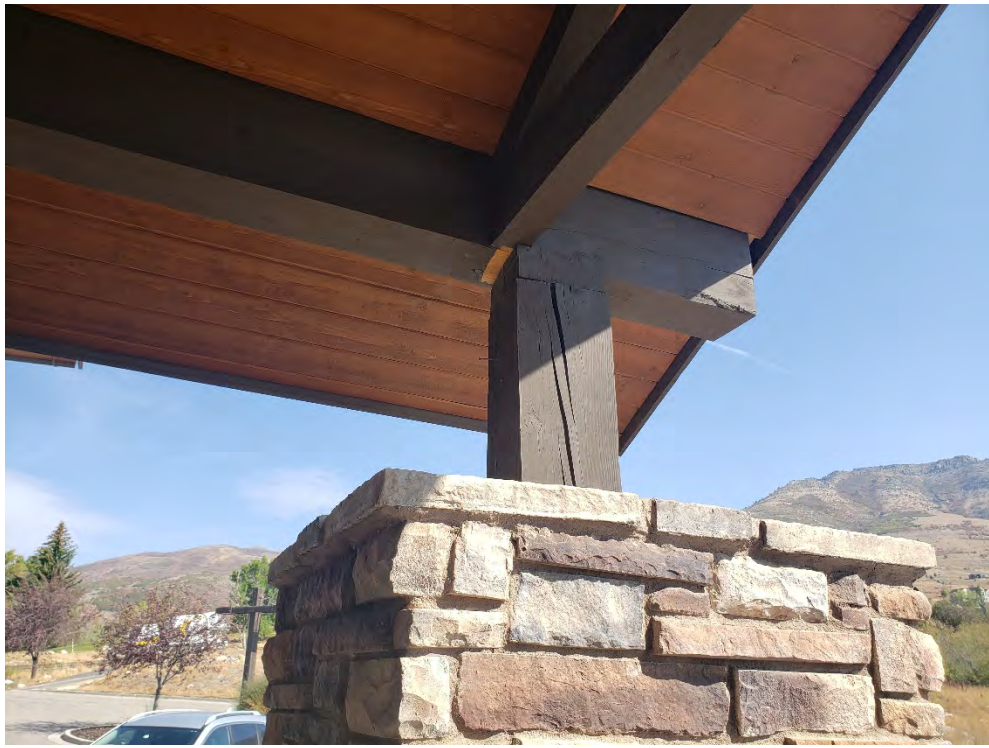
Photo 31. Cracked and displaced roof support.
