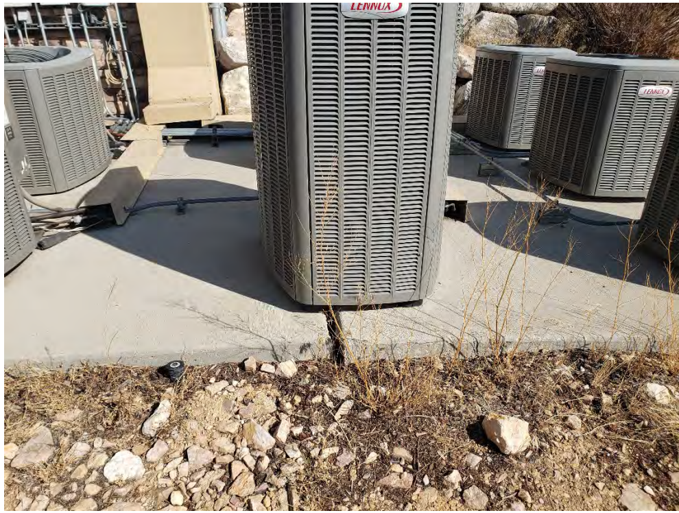
Photo 33. Displacement in AC pad.
