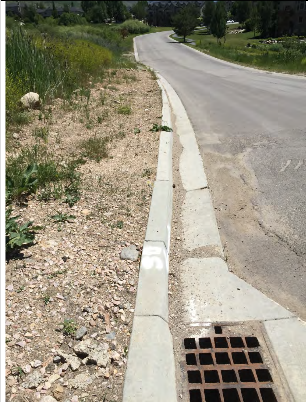
Photo 22. June 2015 UGS site visit. No new displacement at toe.
