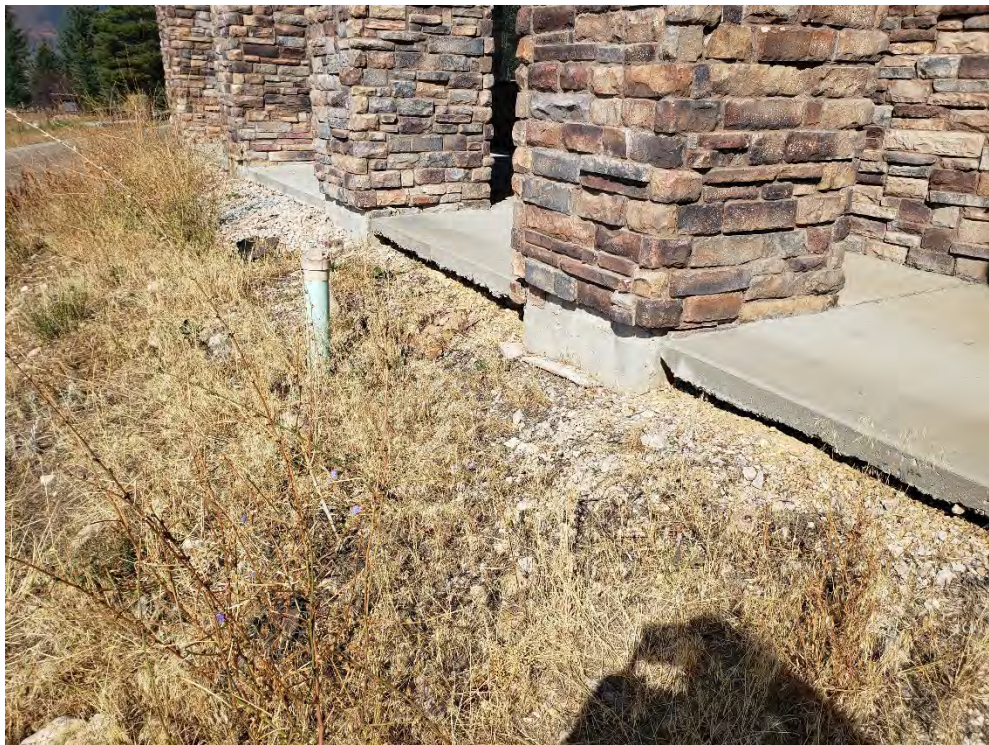
Photo 36. Gap beneath concrete pad on west side of building.
