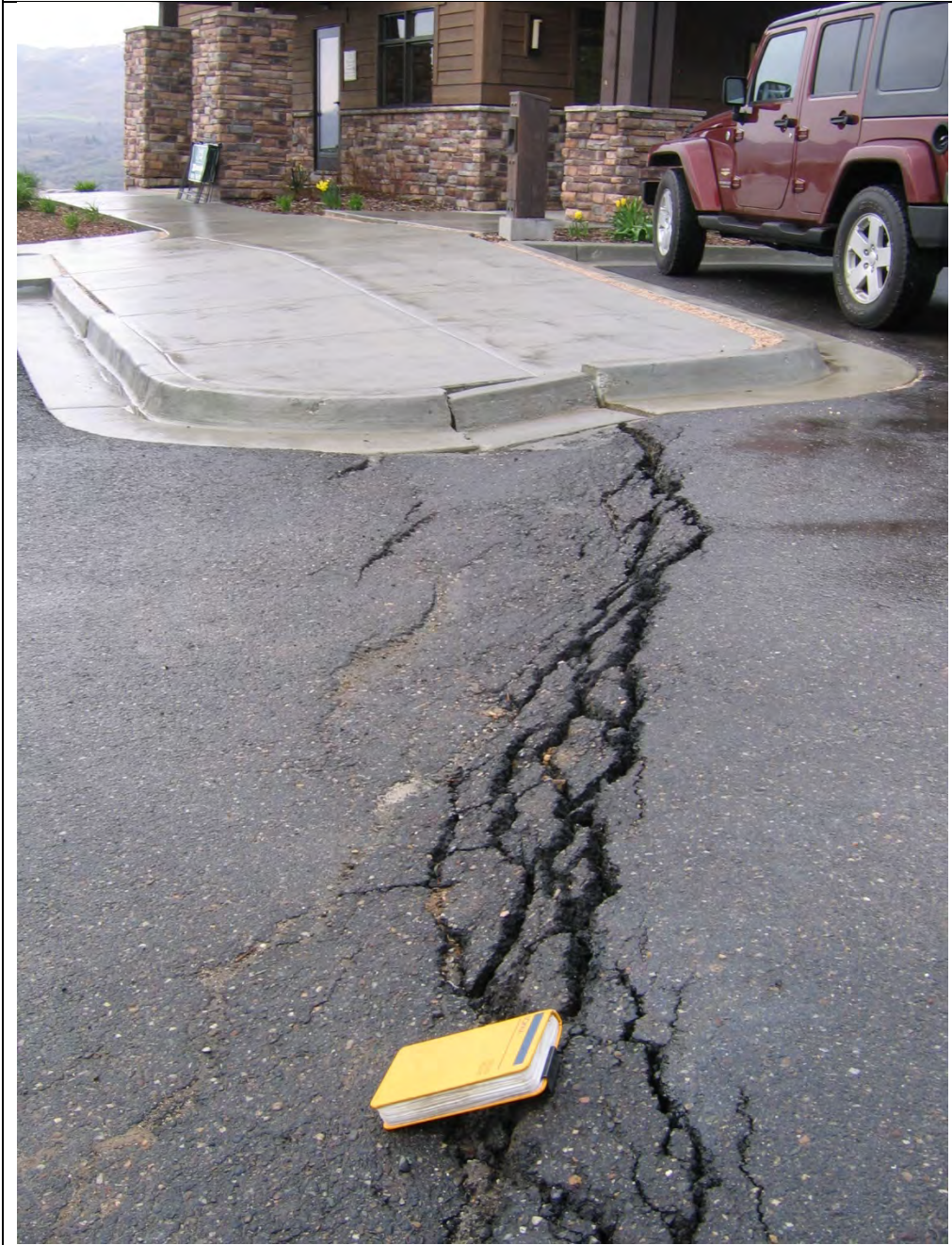
Photo 10. May 2009 UGS site visit. More displacement in parking lot at site.
