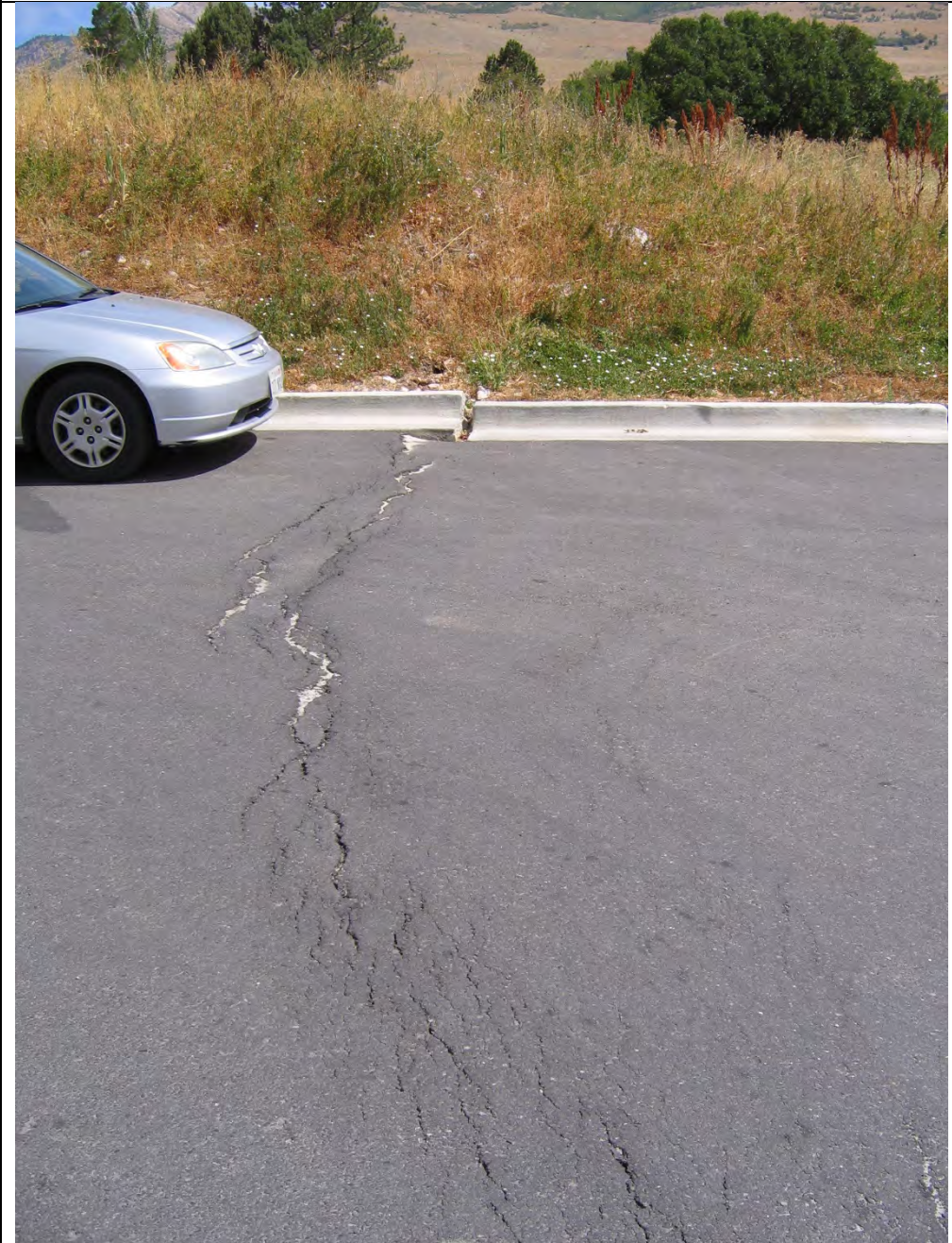
Photo 5. August 2008 UGS site visit. Cracking and displacement in curb and gutter.
