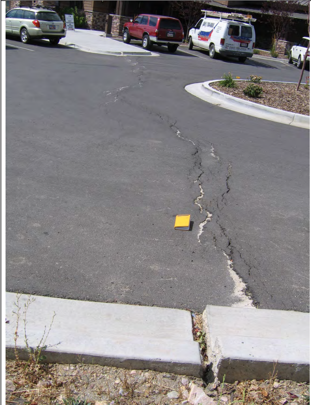
Photo 6. August 2008 UGS site visit. Displacement in parking lot at site.
