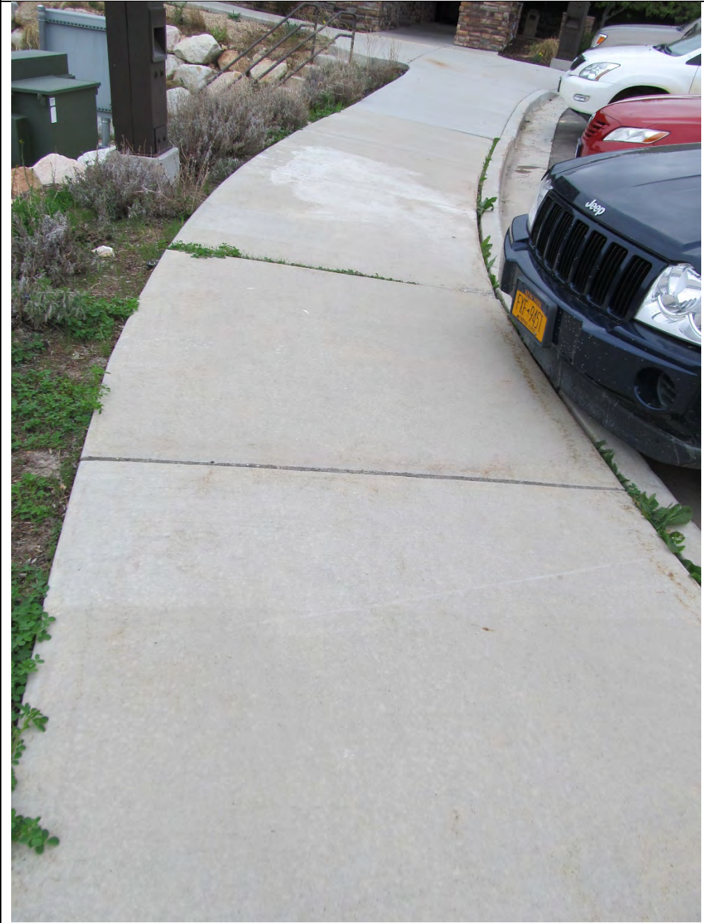
Photo 19. April 2014 UGS site visit. Back tilting in sidewalk at site.
