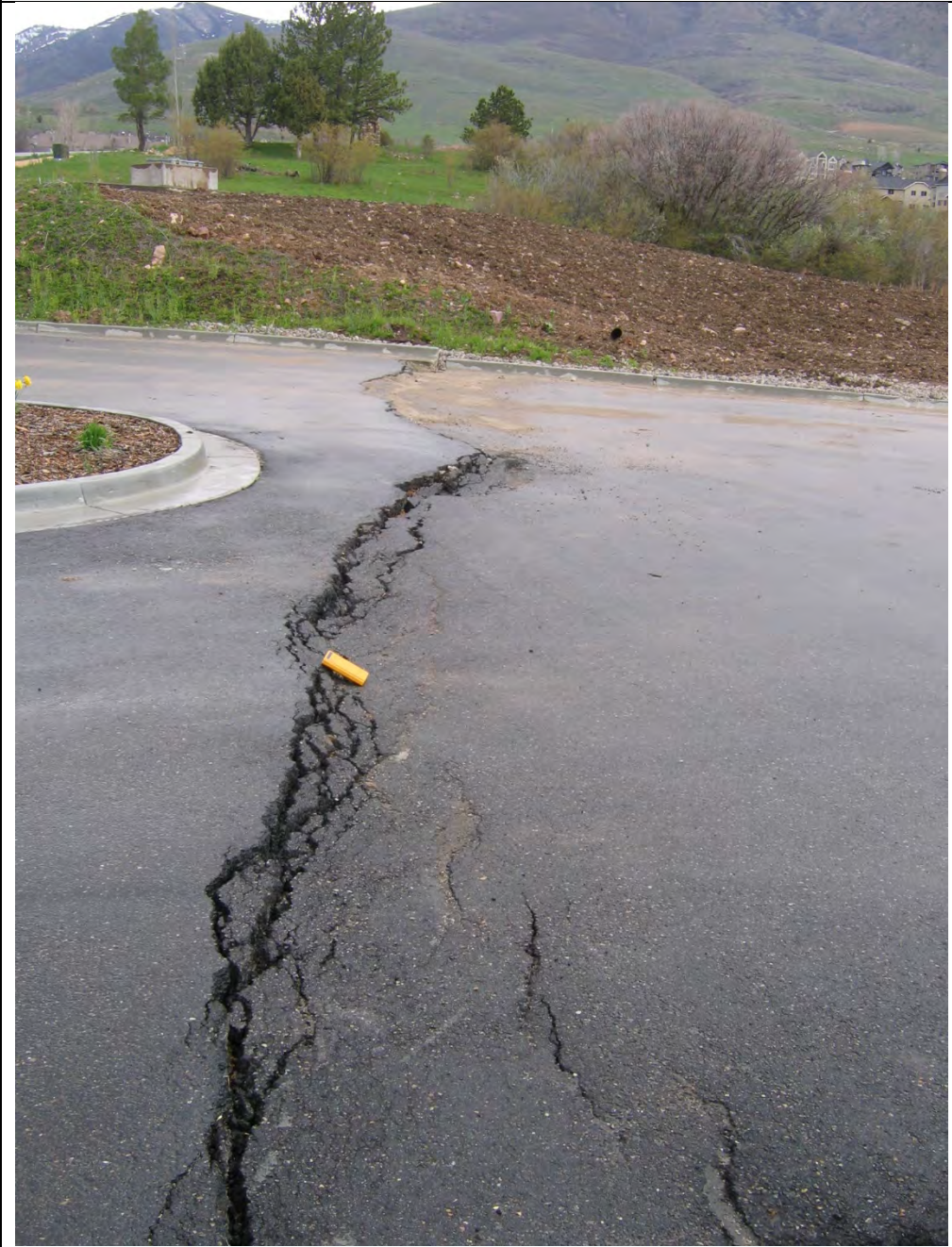
Photo 9. May 2009 UGS site visit. More displacement in parking lot at site.
