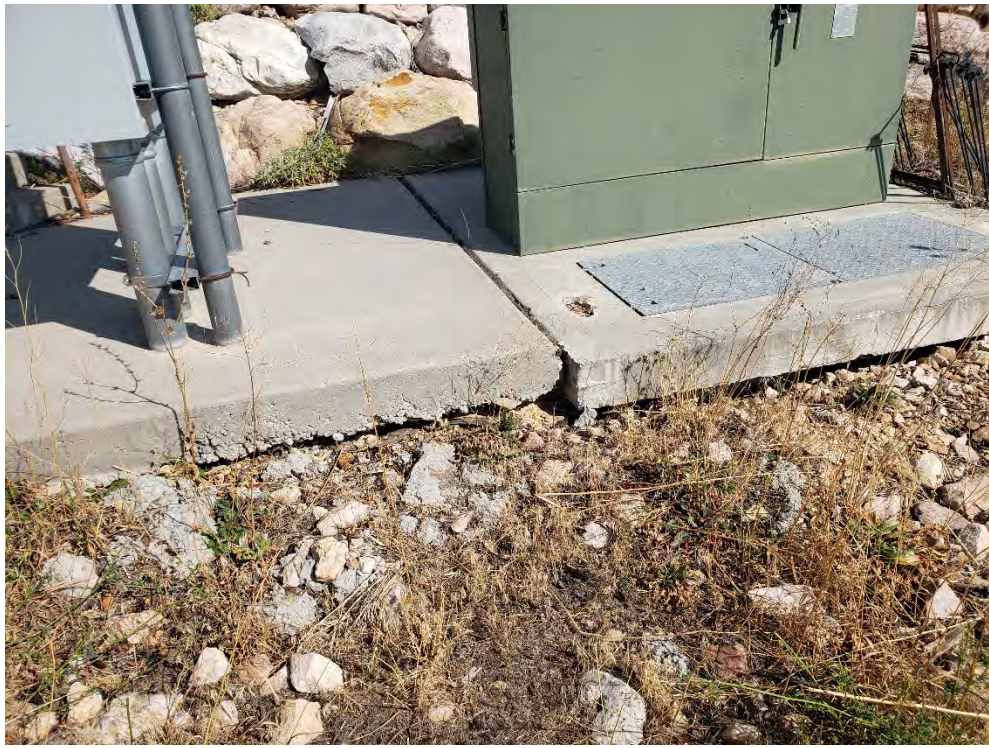
Photo 29. Displacement in transformer pad.
