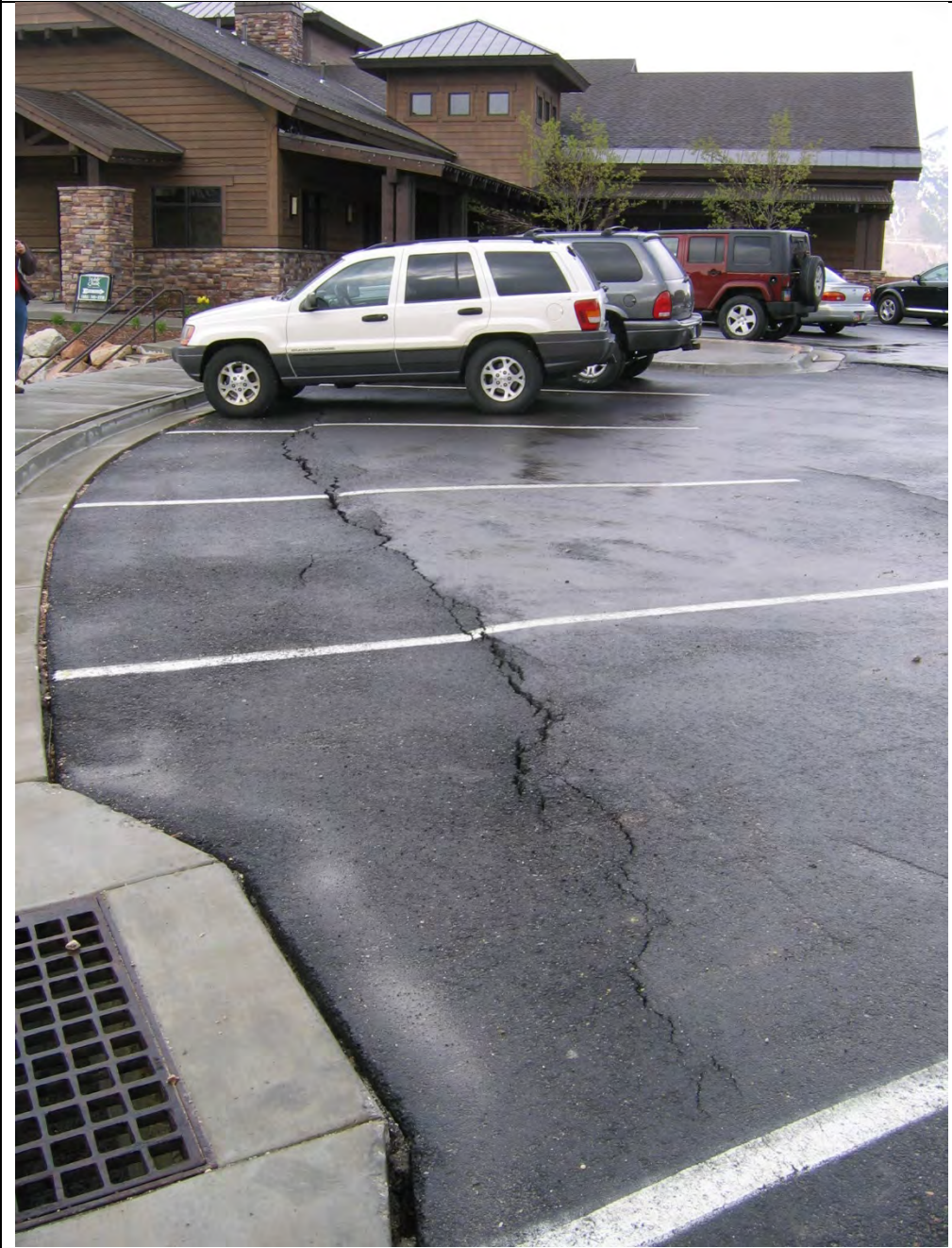
Photo 11. May 2009 UGS site visit. Cracking near storm drain in parking lot.
