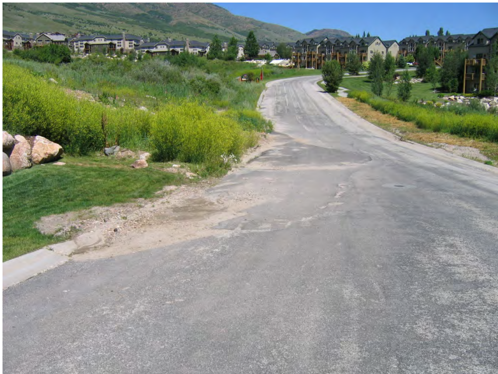
Photo 16. July 2009 UGS site visit. Obvious toe bulge in Moose Hollow Drive.
