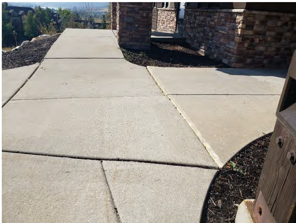
Photo 34. Settlement in sidewalk near entrance, but no concrete cracking.
