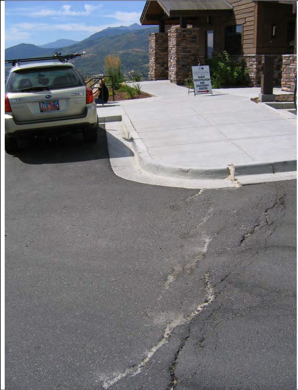
Photo 4. August 2008 UGS site visit. Displacement in side walk and pavement.
