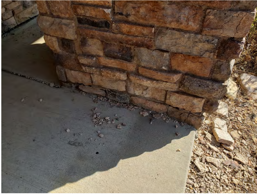
Photo 35. Settlement (tilting) in concrete pad on west side of building.
