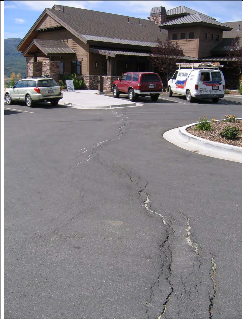
Photo 3. August 2008 UGS site visit. Displacement across parking lot at site.
