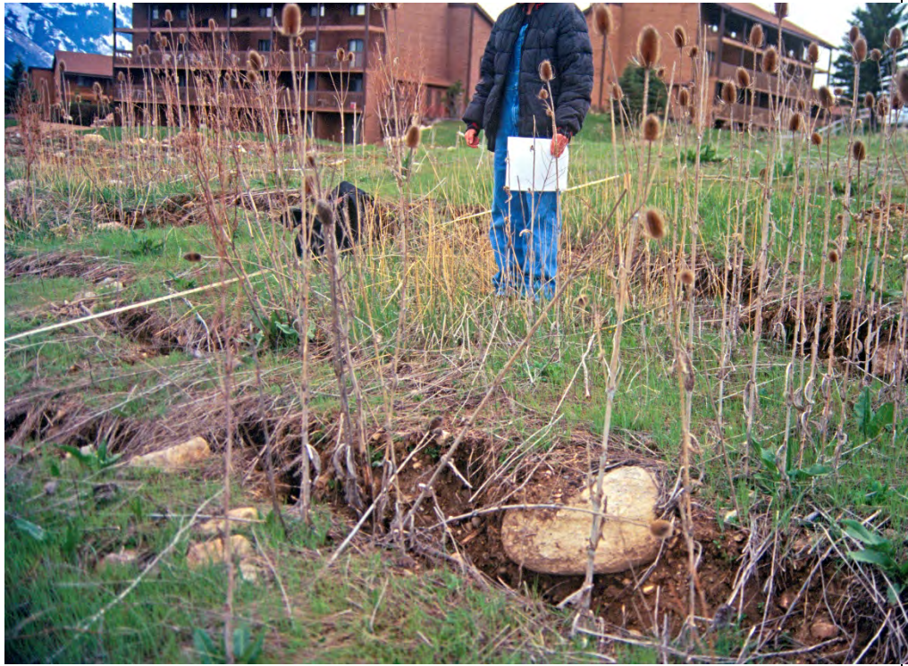
Photo 1. April 1999 UGS site visit. Eden Water Tank Landslide.
