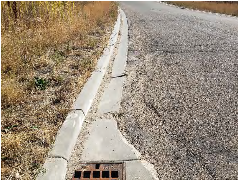
Photo 27. Toe area. No new movement compared to Photo 26.
