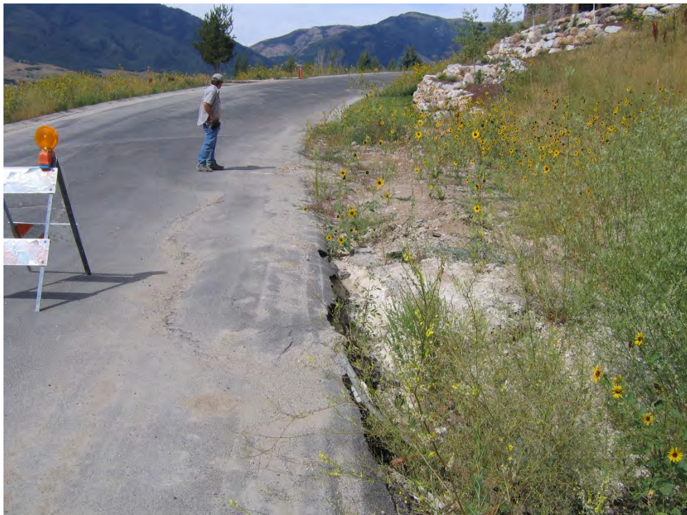
Photo 8. August 2008 UGS site visit. Subtle toe bulge in Moose Hollow Drive.
