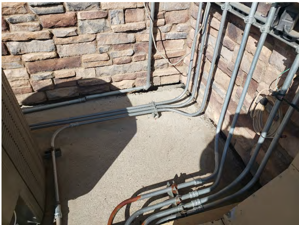
Photo 32. Pull apart between AC pad and building.
