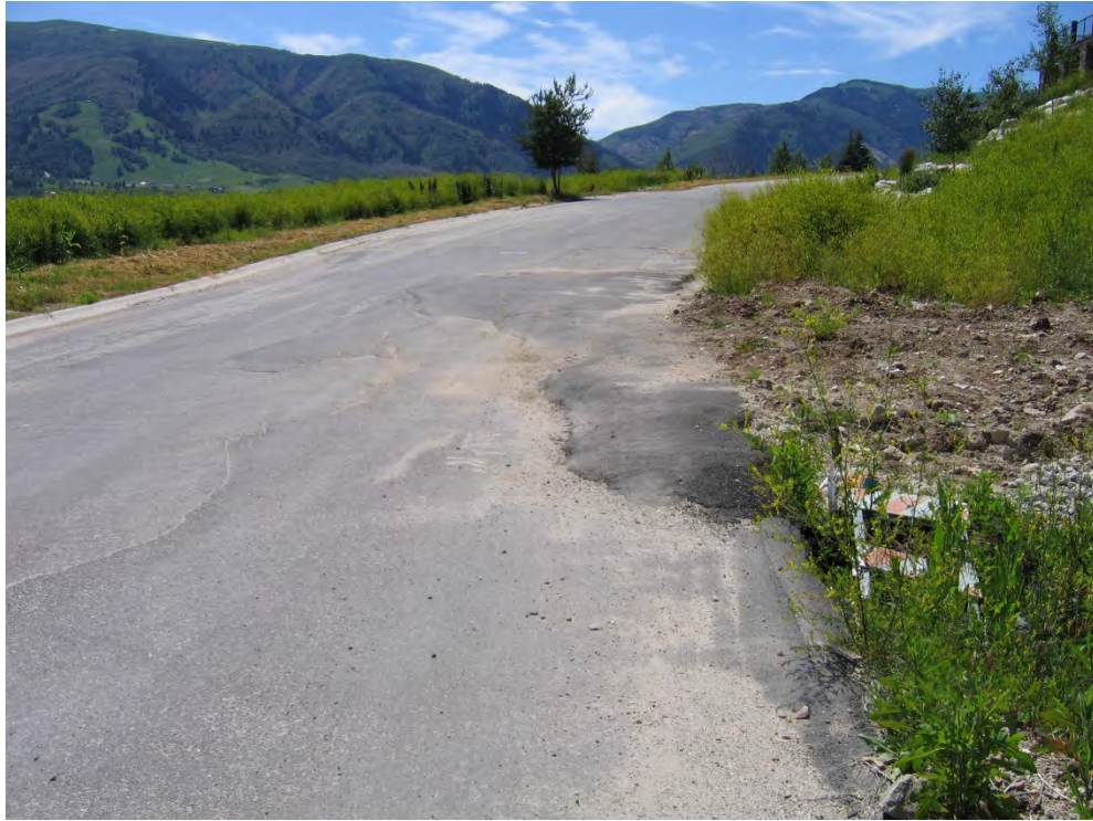
Photo 15. July 2009 UGS site visit. Toe bulge in Moose Hollow Drive.
