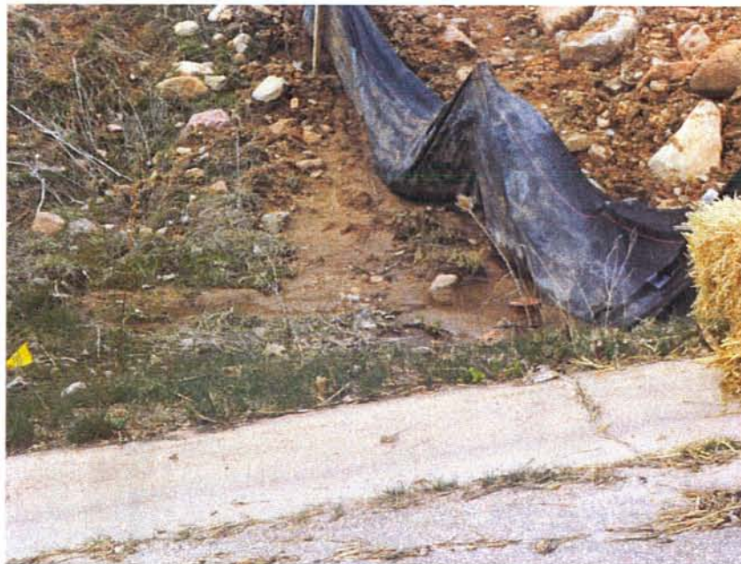
Silt and sediment leaving the site
