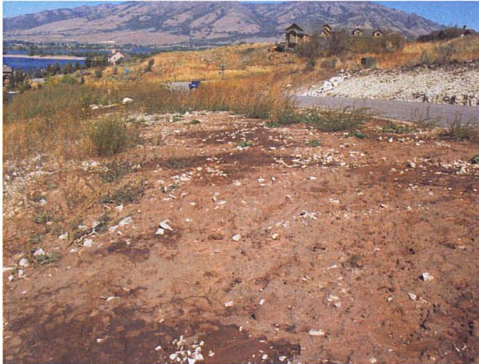
Downhill side of road is not stable
