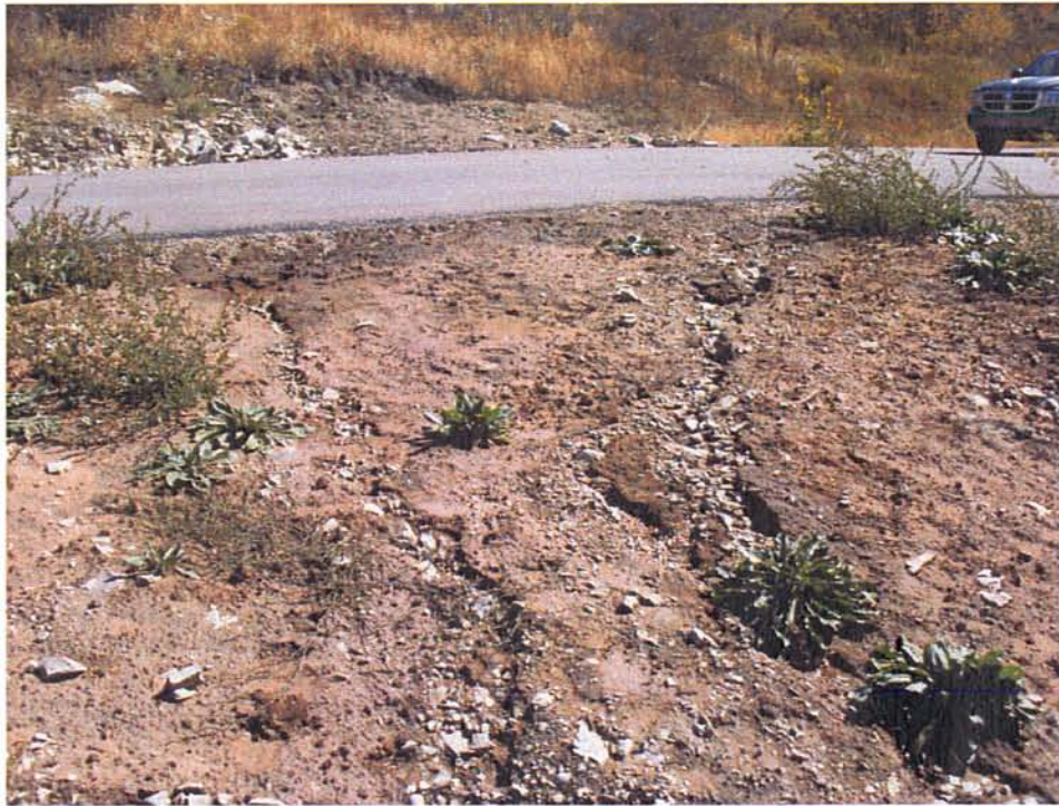
Reels have formed due to the erosion
