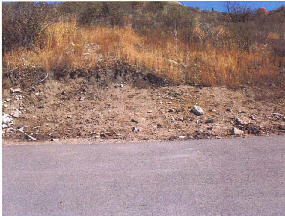
Uphill side of road is not stable
