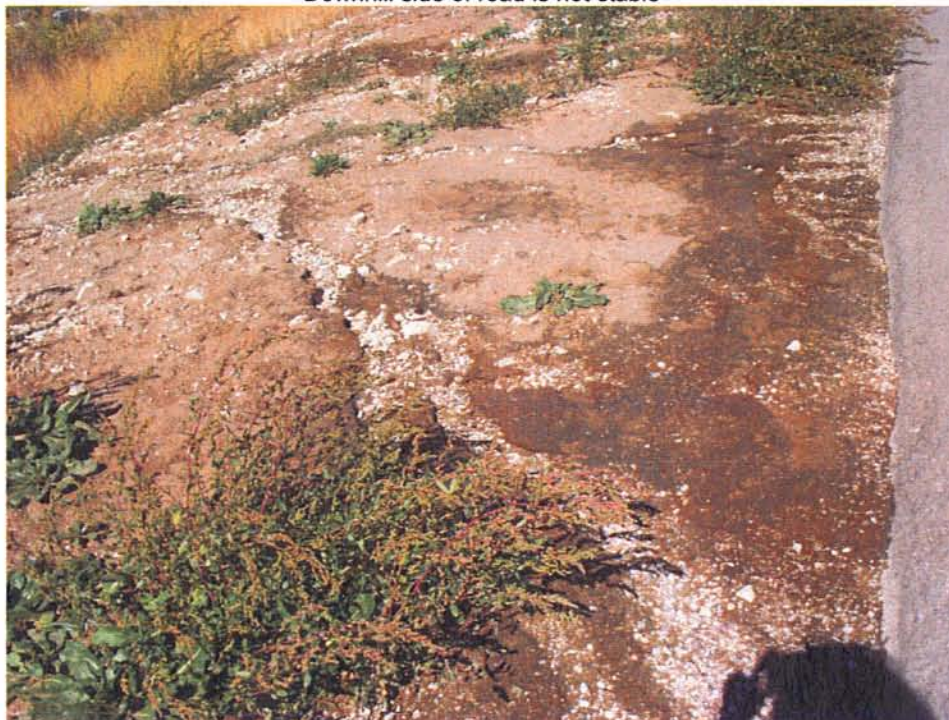
Erosion is evident
