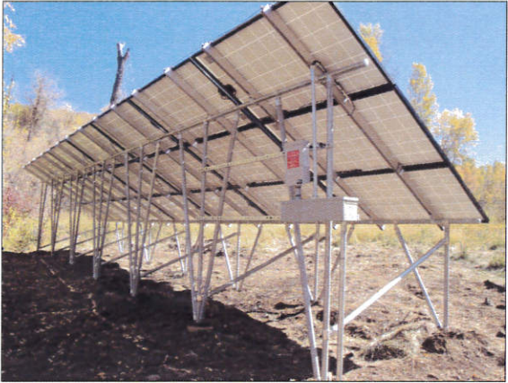
SIMILAR GROUND MOUNT INSTALLED BY GARDNER ENGINEERING AES
